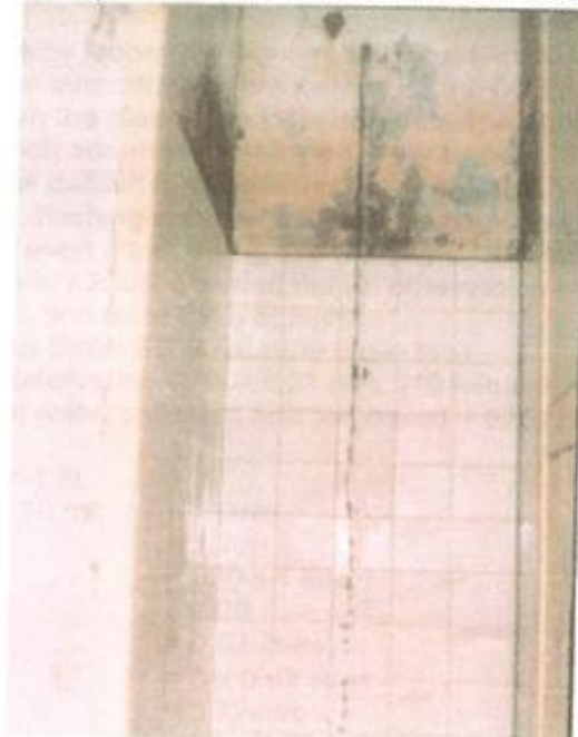
Photograph of running water in the bathroom Block SC B ground floor)
