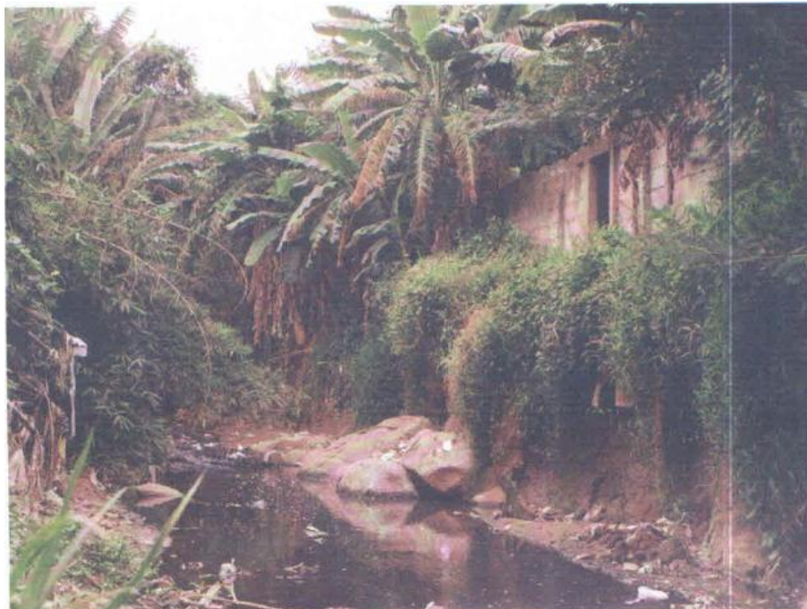
Plate 1: Erosive impact of River Ajilosun at Mofere lower reaches of the river. The building in the picture was excessively elevated due to the pronounced vertical dissection of the river Ajilosun channel. The building, although a bungalow, now appears as a storey building.
